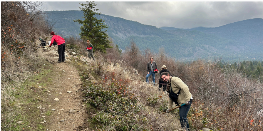
ONA and Wildsight Youth Climate Corps workers roughing the ground along the trail with rakes and spreading native grass seeds just before the first snowfall.
