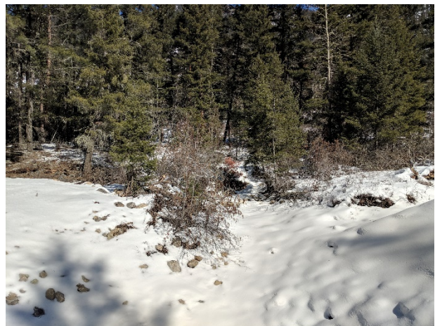
Stop 2: View upstream from replaced culvert, where debris flows occurred with flooding (RL)
