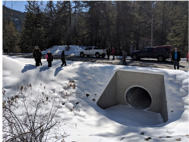
Stop 2: New culvert and headwall installed on upstream side of Hedley Road (CM)
