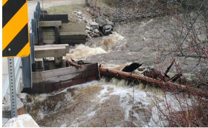
Figure 5: Debris blockage upstream of a bridge on Princeton-Summerland Road, 2017 (Source: RDOS).
