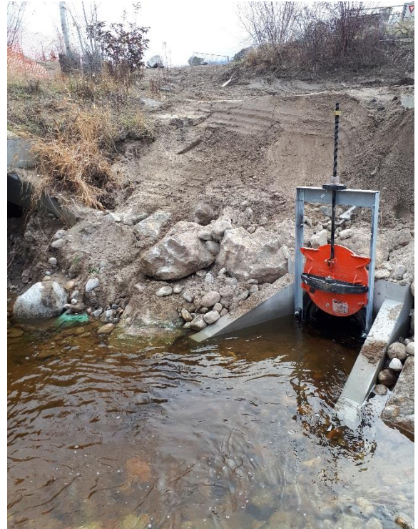
Bypass system inlet
