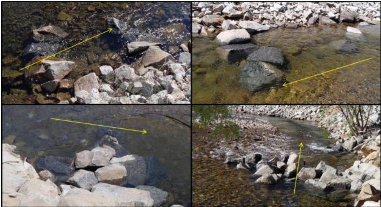
Figure 8. Examples of rock groyne fish habitat structures created to deflect the thalweg at low flows from the rip-rap bank and provide fish habitat at Pass Creek, flow direction indicated with yellow arrow (all pictures taken by Evan Smith, Okanagan Nation Alliance, July 2015).
