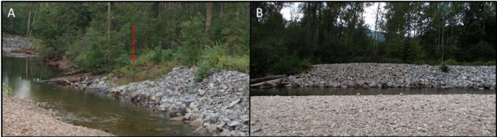
Figure 5. (A) Upstream view of Section 1 (indicated by the red arrow) before repairs were made. (B) View of Section 1 from across the stream after repairs were made pictures taken by Evan Smith, Okanagan Nation Alliance, July 2015).
