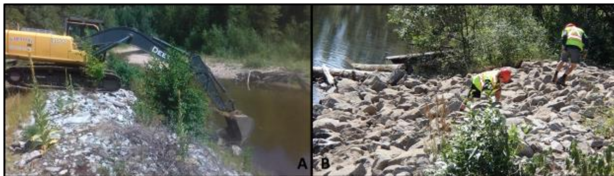
Figure 4. (a) Excavator placing rip-rap on the right bank of Pass Creek at the Pass Creek Regional Exhibition. (b) Regional District of the Central Kootenay employees placing smaller rock in holes to cover all geotextile fabric and spaces in the rip-rap (pictures taken by Evan Smith, Okanagan Nation Alliance, July 2015).
